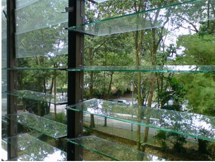
Figure 6: Automatic Louvered Windows
